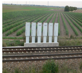
Monitoring system near Vienna consisting of six chained portals.
